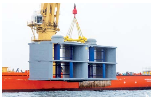
OceanQuest 1MW tidal turbine immersed at Paimpol Bréhat in April 2019
