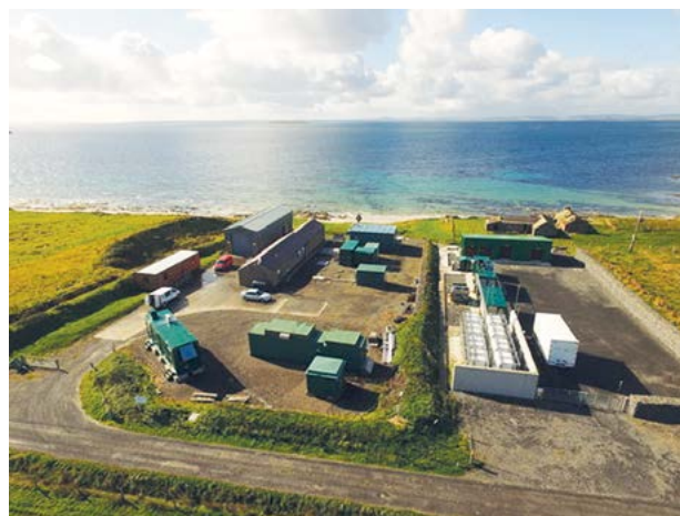
EMEC Caldale substation and hydrogen plant (Source: EMEC)
